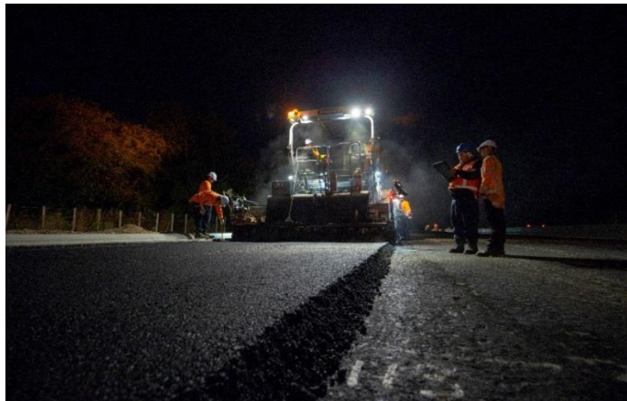
Night works from 24-27 June will allow road crews to complete the new intersection opposite Bollard Road.
