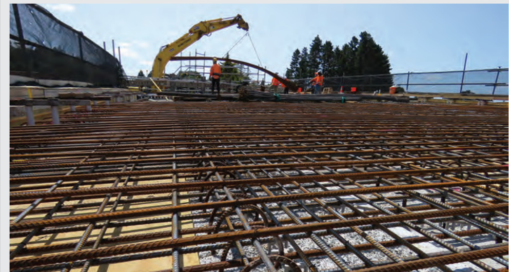
The Cambridge Road bridge deck is under construction. Final excavation of the expressway is now advanced. A raised embankment has been constructed across the East West Gully. This will carry the new link road from Cherry Lane, across the East West Link Bridge and across the gully to Birchwood Lane. The new road layout for Bollard Road and Cambridge Road is under construction.
