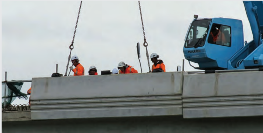
Final barrier construction and service relocations are under way on this bridge which crosses the East Coast Main Trunk Rail Line and Ruakura Road.
