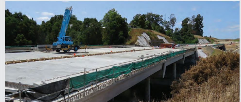
These bridges are nearing completion. The decks are now complete, along with the end walls and settlement slabs. Placement of bridge barriers will commence shortly. Construction vehicles can now travel across these bridges for the first time.
