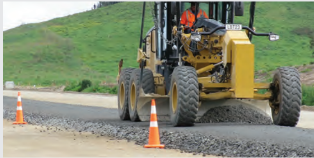
The first layer of Hi-Lab road rock is being laid, cement stabilised and compacted at the tie-in to the Ngaruawahia section of the Waikato Expressway, immediately north of Lake Road.
