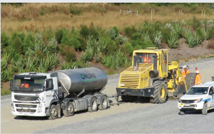
The first layer of Hi-Lab road rock now extends 8km from Lake Road in the north to the Puketaha Road Bridge, and will continue north to south. The Puketaha Bridge is complete.
