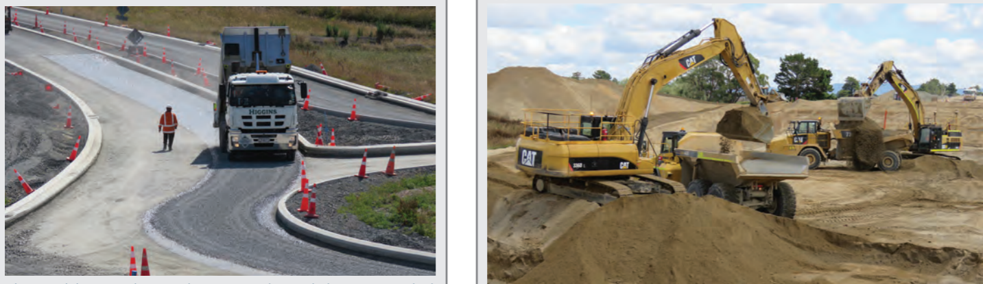
Rock and sand placed on top of Powells Road has been removed. Ground improvements are about to begin for the Powell's Road Underpass. This will protect the underpass structure from liquefaction in earthquakes.
