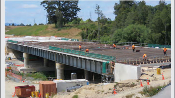
The steel bridge structure is complete. 600 concrete panels have been laid on top. These are now being tied together by a series of concrete pours to form the deck. Construction of this bridge is expected to be complete in mid 2020.
