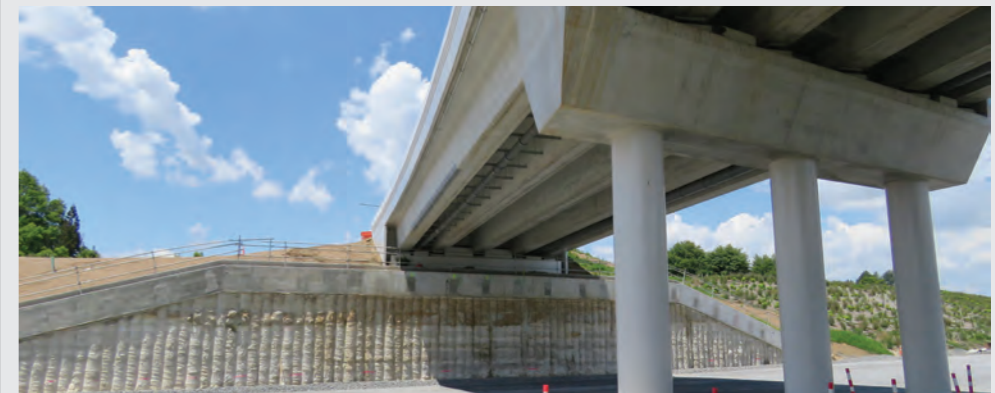
Before the beams were placed on the East West Link Bridge, a wall made from intersecting concrete piles was created under the eastern end of the bridge. The wall was tied back to a large concrete anchor to reinforce it, then the ground on the opposite side was excavated out to form the retaining wall. This is called a secant wall. The piles are formed by a large auger that drills a series of deep holes and backfills them with concrete.
