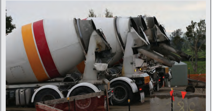
The underpass structure is almost complete. Eighty concrete trucks supplied 500 cubic metres of concrete on 3 February to pour the roof of the underpass. Sand is now being placed and compacted either side of the underpass to take the expressway over the top.
