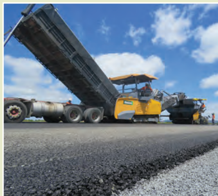
A truck tips asphalt into the shuttle buggy, which sends it on by conveyor to the paver.
