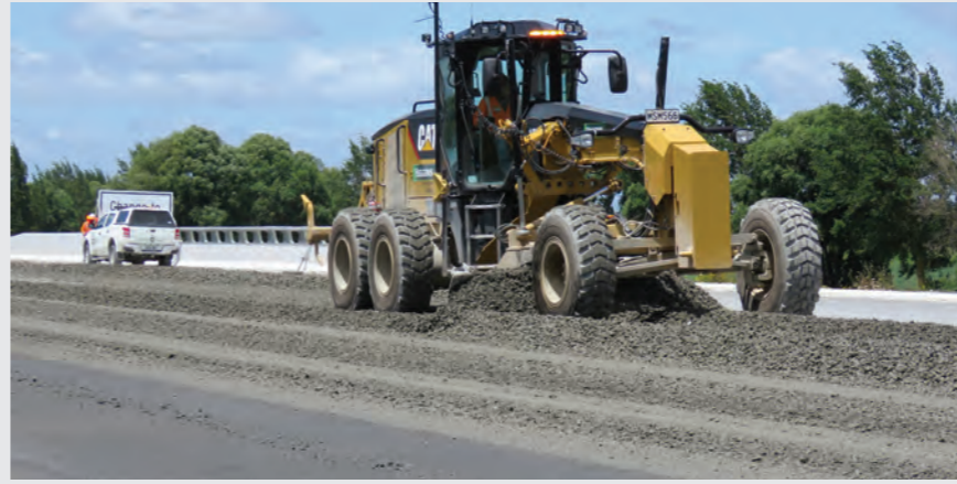
Prime coating and chip sealing is progressing south. Pavement rock is being blended and supplied from our blending plant near the Puketaha Road Bridge.
