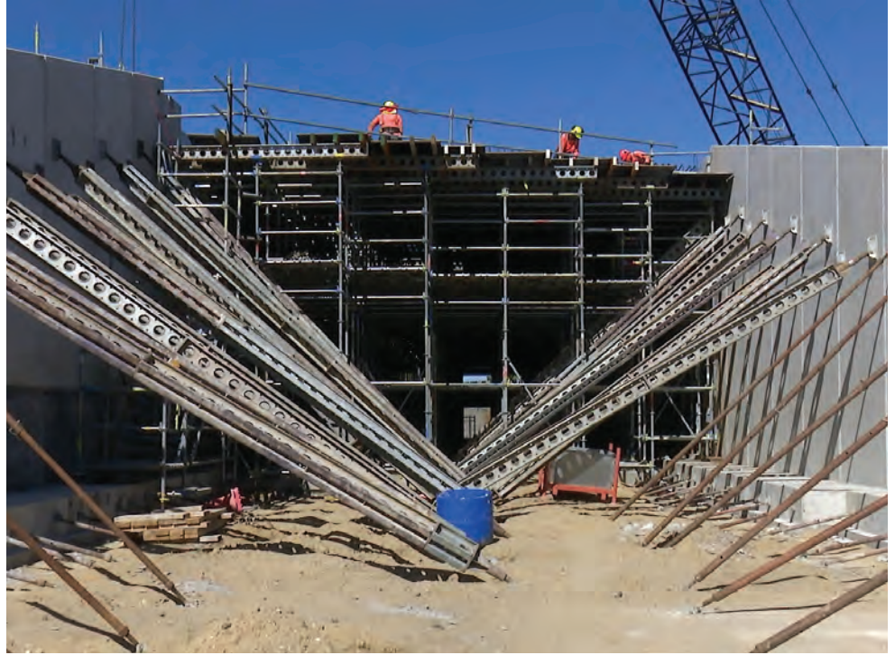
Braces and scaffolding provide support until the deck is poured on top.
