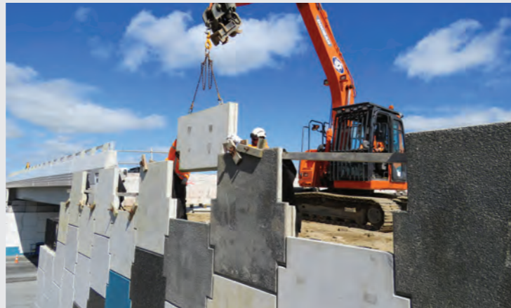
The bridge abutments have been completed. Planting and landscaping is progressing. Construction of the link to Resolution Drive has recommenced. Chip sealing of the main expressway is complete.
