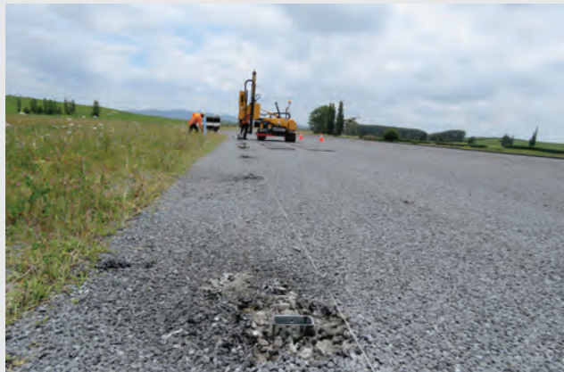
Flexible barriers are being installed. First the sleeves are driven into the pavement. The posts that hold the wire rope fit inside the sleeves. Across the project, 77km of flexible wire rope barrier is being installed.
