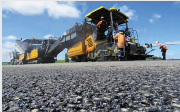
The final asphalt is being laid north to south from Lake Road. A northbound off-ramp from the Ngaruawahia Section to Lake Road is under construction. Work has begun to tie in the lanes on the Hamilton Section lanes with the lanes on the Ngaruawahia Section.
