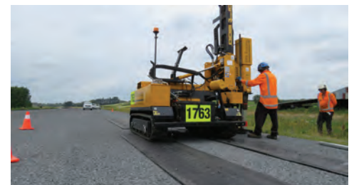
The hydraulic ram unit drives sleeves into the pavement to hold the barrier posts.
