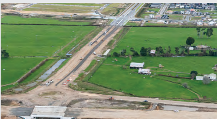
The new road layout for Greenhill Road is well advanced. Drainage is complete along the Pardoa Boulevard extension, and road construction to the Greenhill Interchange is under way. Greenhill Road east of the interchange will connect with Pardoa Boulevard.
