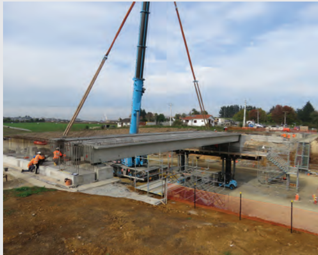
The beams have been placed and the deck poured on top. This bridge will take Horsham Downs Road over the expressway. Completion later this year will mean Horsham Downs Road can be reopened to traffic.
