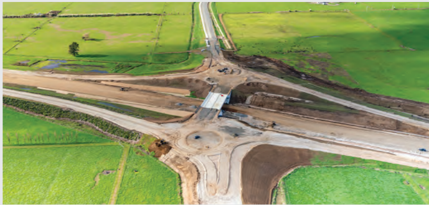
The interchange bridge is completed. The Ruakura Road East connection to Morrinsville Road is largely complete. Design for the Ruakura Road West connection to Silverdale Road is currently being developed.
