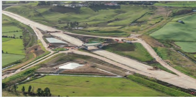
Beams have been placed on the bridge. Permanent wetlands to treat run-off from the road have been shaped and planted.
