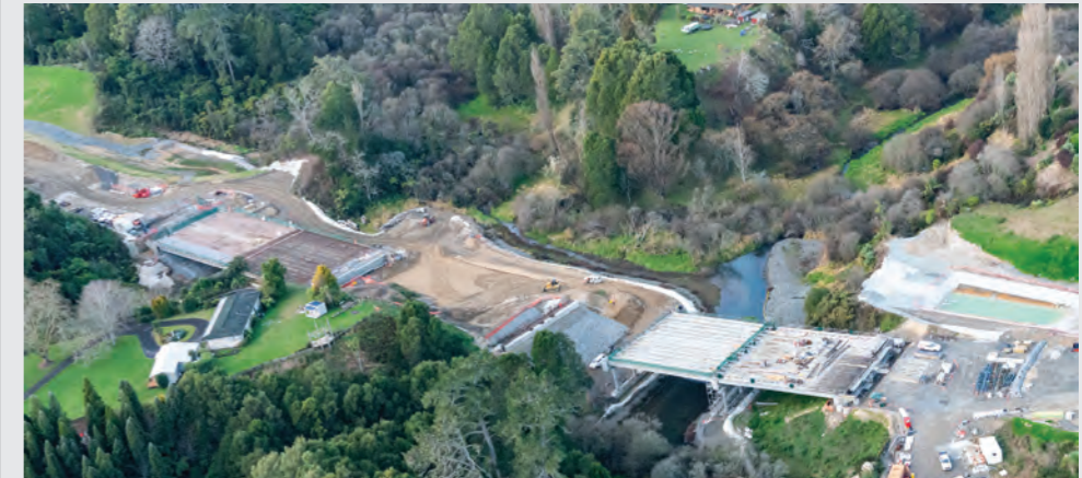
The last beams are about to be delivered and installed, followed progressively by concrete deck pours. Construction of both bridges is now well advanced.
