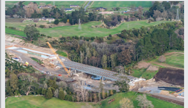
Steel beam installation is now complete. Construction of the concrete deck has begun.
