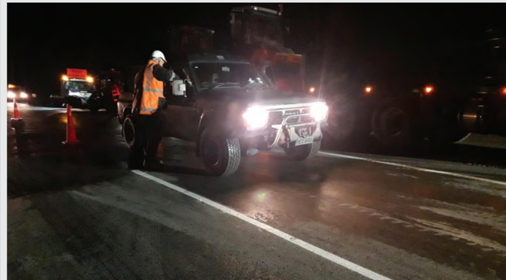
The first vehicle travels over new SH1 lanes running under the East West Link Bridge on 8 July. A new temporary intersection is in place opposite Bollard Road for residents in Bollard Road, Cherry Lane and the section of Cambridge Road in between. This will remain until the project is complete.
