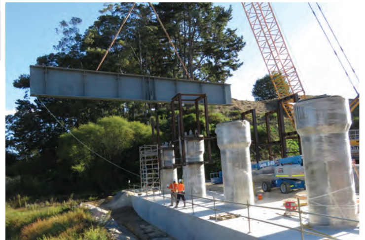
The first bridge beam is lifted into place on the Mangaonua Bridge.
