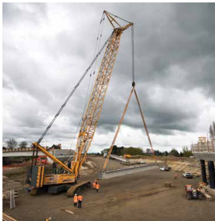
A 300-tonne crane lifts a beam into place at the East West Link Bridge
