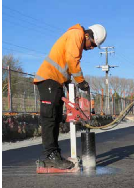
When new asphalt is laid and compacted, core samples are drilled every 50m for testing.
