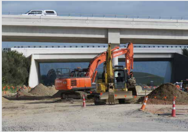
The Hi-Lab blending plant has been relocated from Lake Road to a new base at Puketaha. Drainage installation continues.
