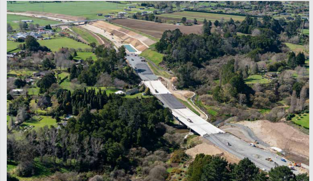
Both bridges are now complete. Drainage installation continues. Preload material has been placed to promote settlement at the bridge approaches.
