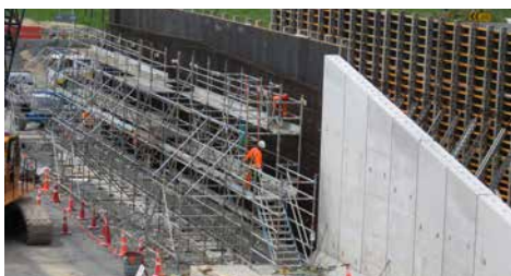
The main walls for the underpass are being formed and poured on site.
