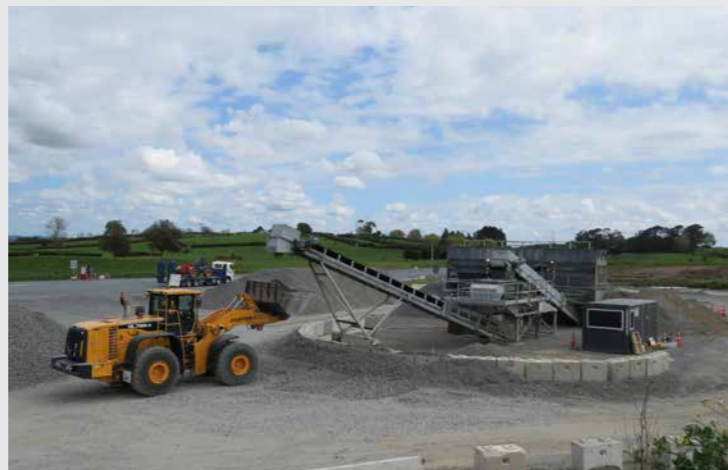
Production of our Hi-Lab rock blend has resumed at the project's relocatable blending plant, now sited near Puketaha Road.
