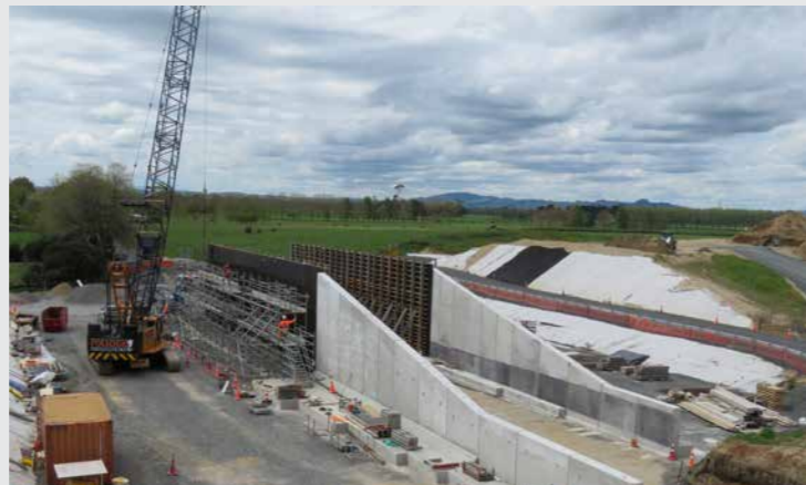
The main walls and western wingwalls of the box culvert underpass are now complete. Construction continues.
