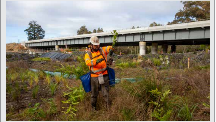
Bridge construction is complete. Gully restoration planting is almost complete. Installation of permanent treatment swales and removal of sedimentation ponds is about to begin.
