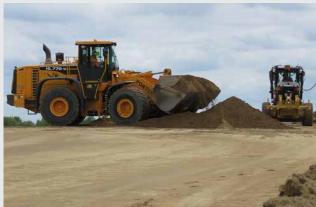
Layers of compacted sand are being prepared and tested in preparation for pavement construction. Chip seal repairs have been carried out on the local road connections.
