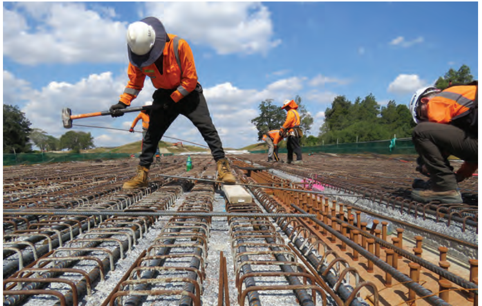
Reinforcing steel is placed and tied off before the final deck pour at the Mangaonua Bridge near SH26 Morrinsville Road.
