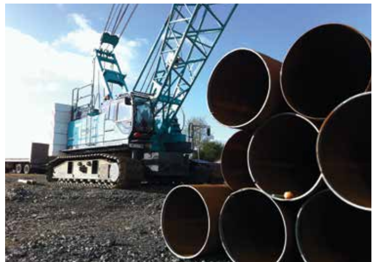
Pile casings ready to be driven by our piling crane at the Ruakura Rail Overbridge.
